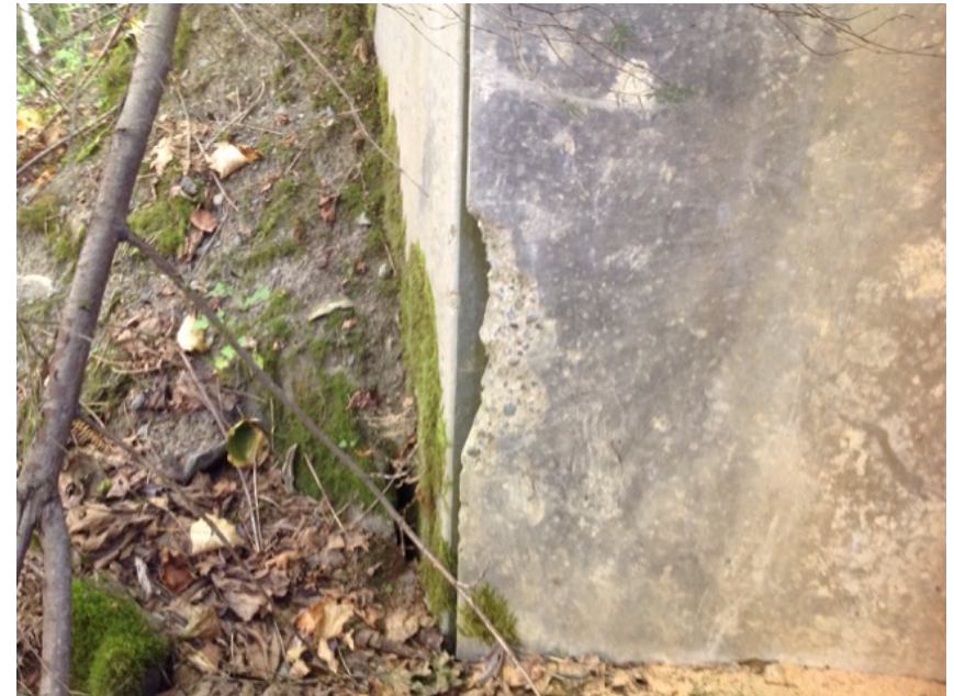
minor damage to concrete ballast wall
