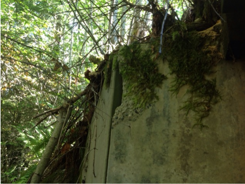
minor damage to ballast wall
